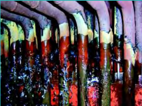
Boiler tube failure
