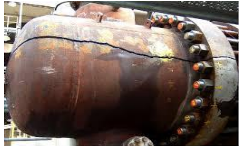
Secondary damage caused by HTHA failure
