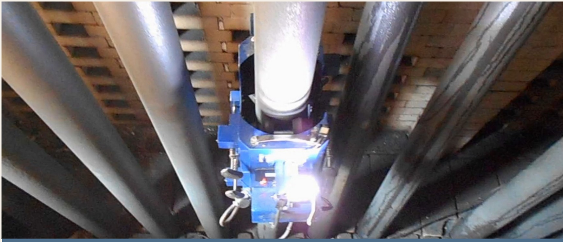
ARTiS inside the furnace box
