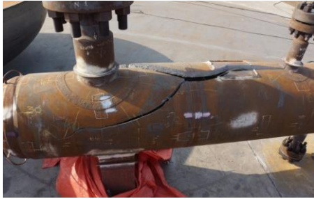
Brittle Failure / Low Temperature
